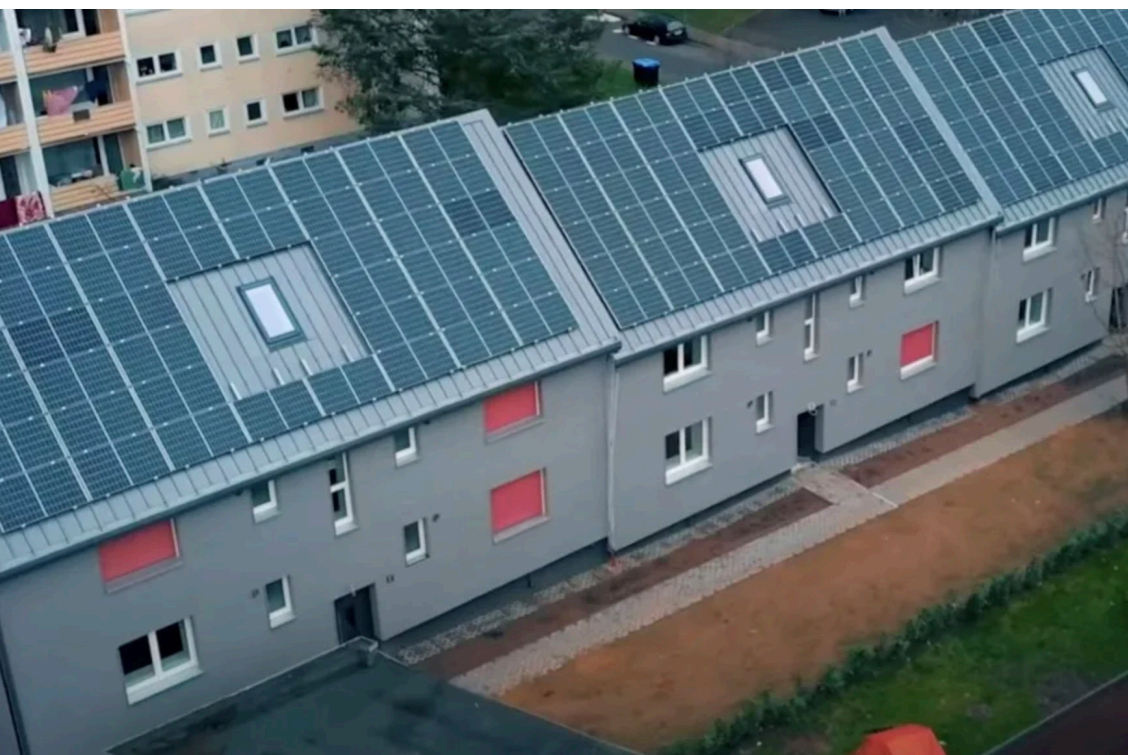
Ecworks carbon neutral prefabricated facades and roof panels installed at project site.
